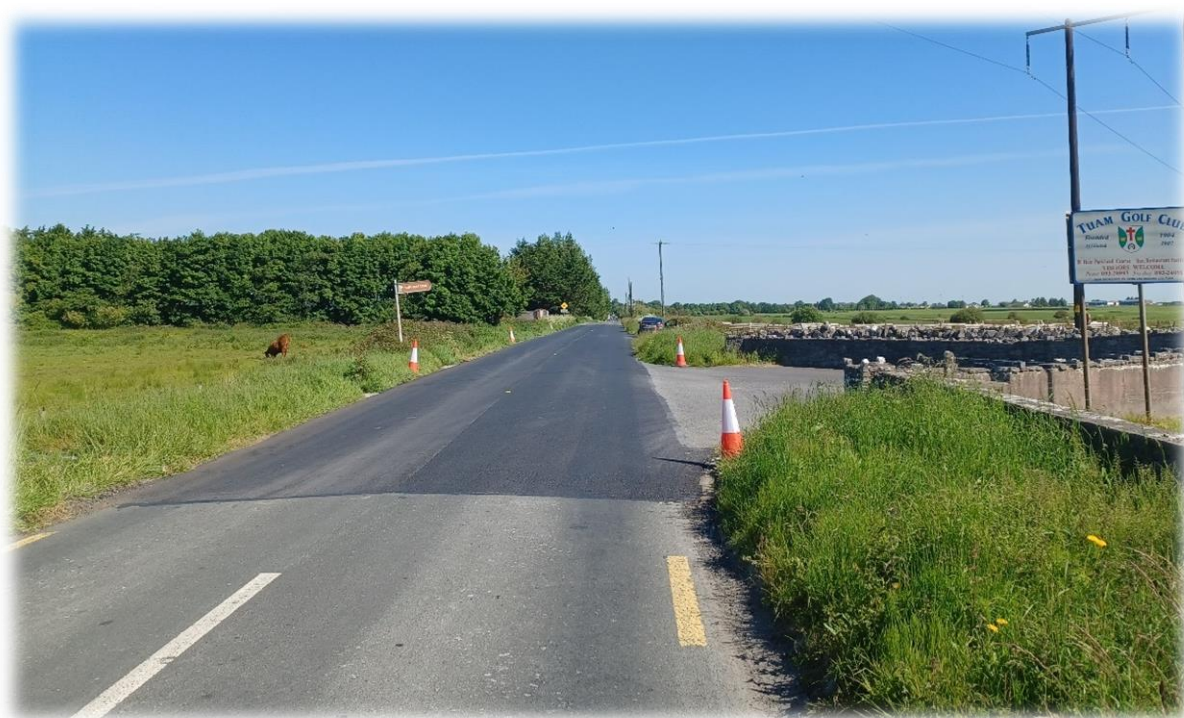
NEW OVERLAY ON THE ATHENRY ROAD, AT TUAM GOLF CLUB, SURFACE DRESSING TO FOLLOW THIS WEEK.
