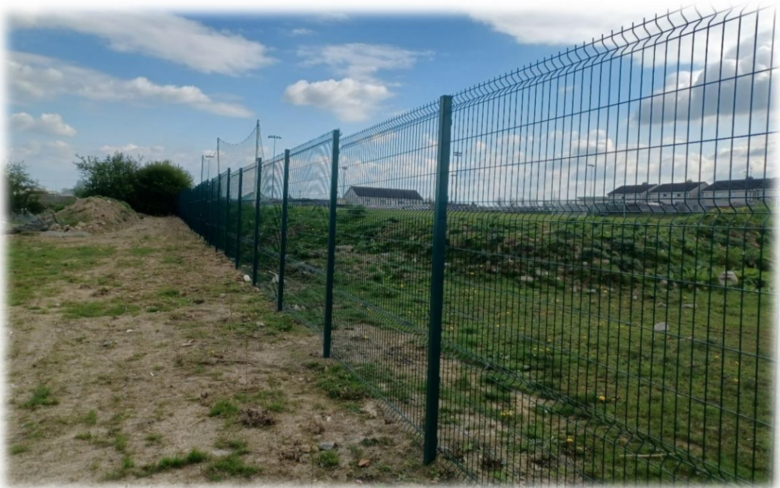
THIS IS A RECENT PALISADE FENCE THAT WE ERECTED AT THE ALLOTMENTS IN PARKMORE IN TUAM. THIS FENCING ENSURES THE SECURITY OF THIS IMPORTANT COMMUNAL PUBLIC PLANTING AREA.
